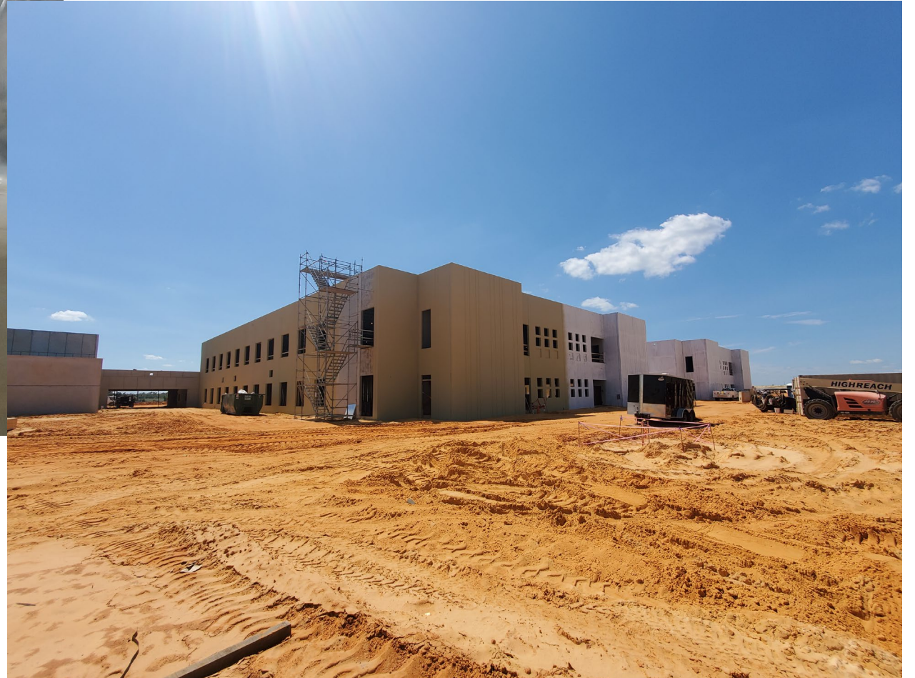
Below is prime paint and texture coating on Building 5 tilt panels from NE looking SW
