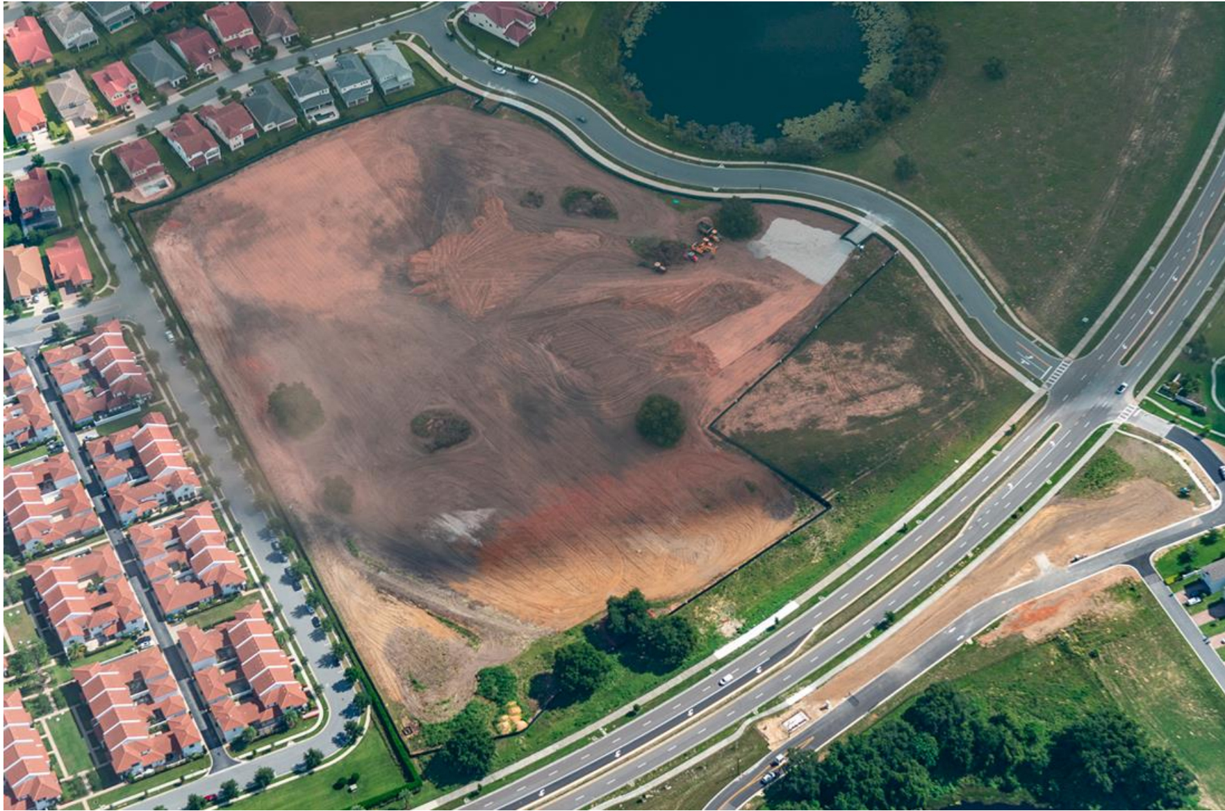
July 2021 – Site 114-E-W-4 : Site Clearing, Construction Entrance and Perimeter Storm Best Management Practices Set
