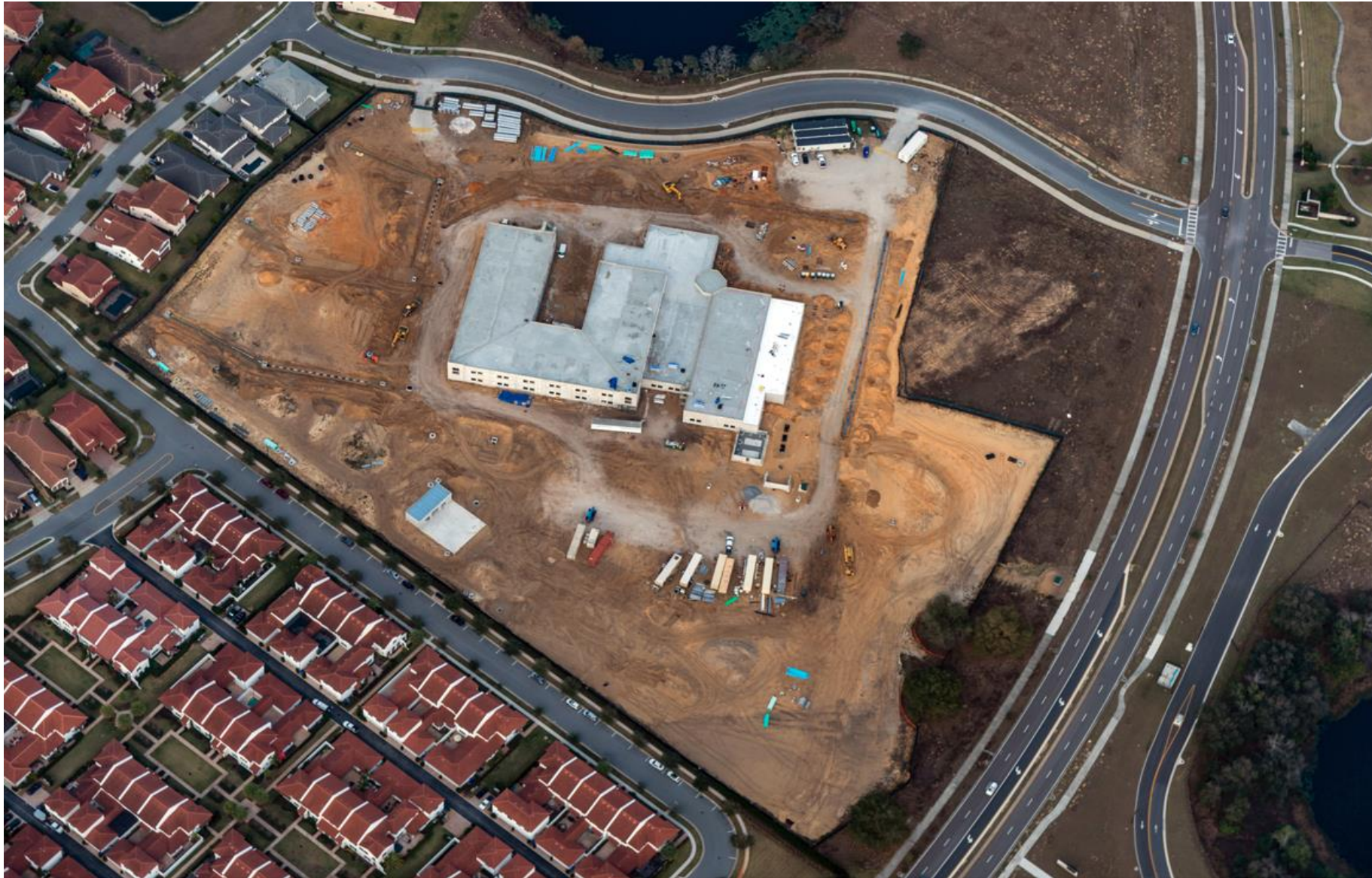
February 2022 – Site 114-E-W-4 : Install Interior Framing and Overhead Mechanical, Electrical and Plumbing. Civil Started
